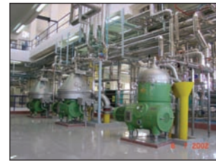
A piping network in an industrial facility.
